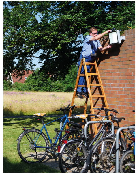
The lighting on the campus has been upgraded to LED technology
